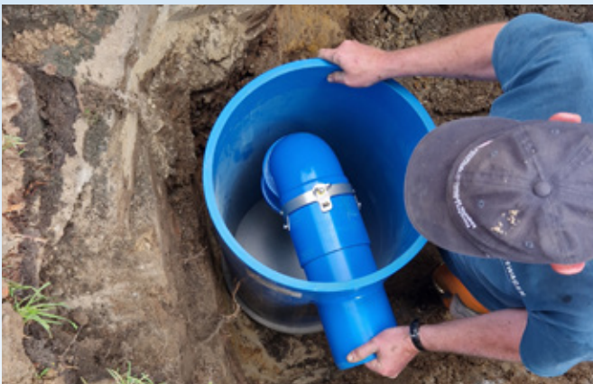
Funke Dry Trap Gully with Funke Quick Coupling® and submerged pipe bend
