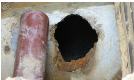
Typical damage pattern: Broken and dimensionally unstable openings.
